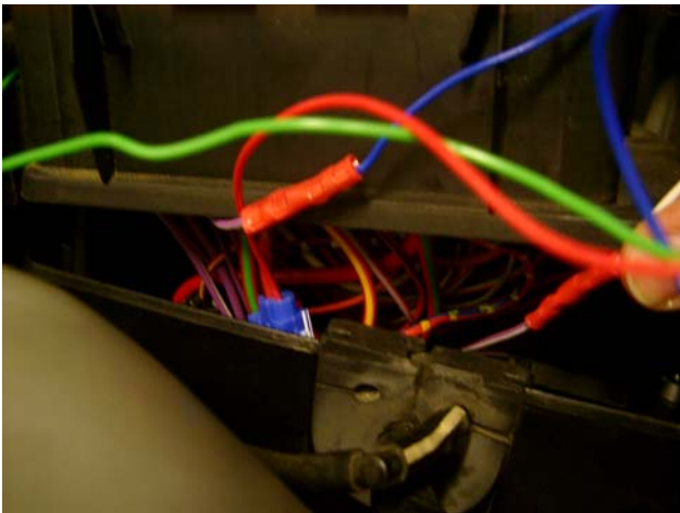
Picture 9: Connection of relays
